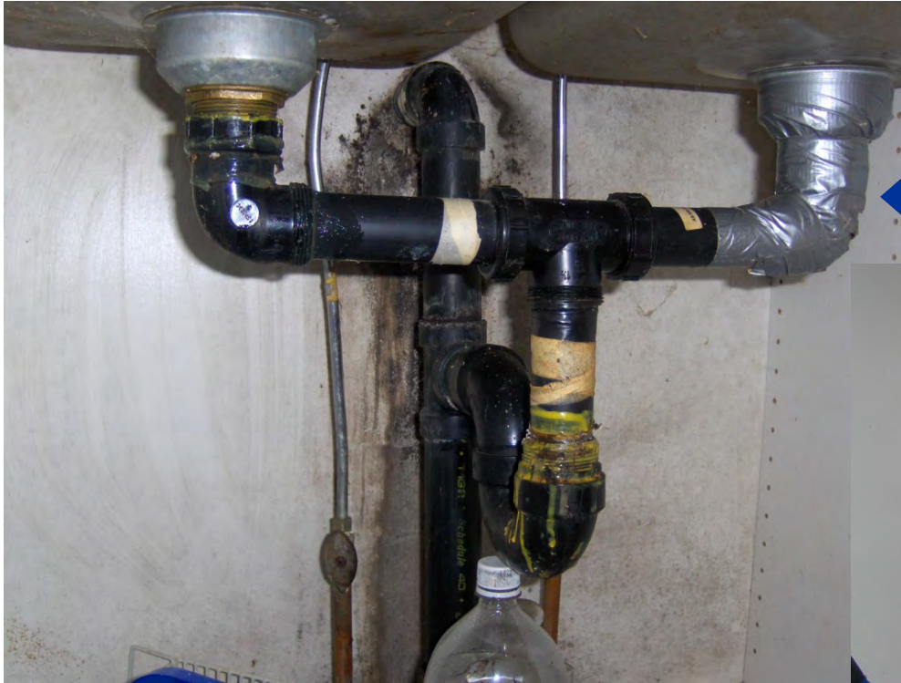
Under counter plumbing
